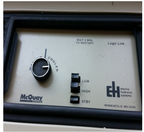
Perimeter units with manual controls
