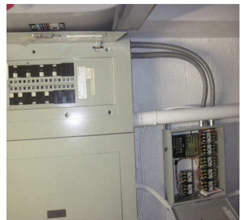
Breaker panel—now with breaker level controls
