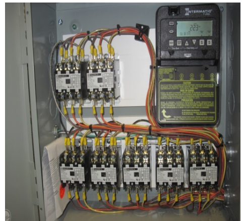
Breaker level controls with a timeclock
